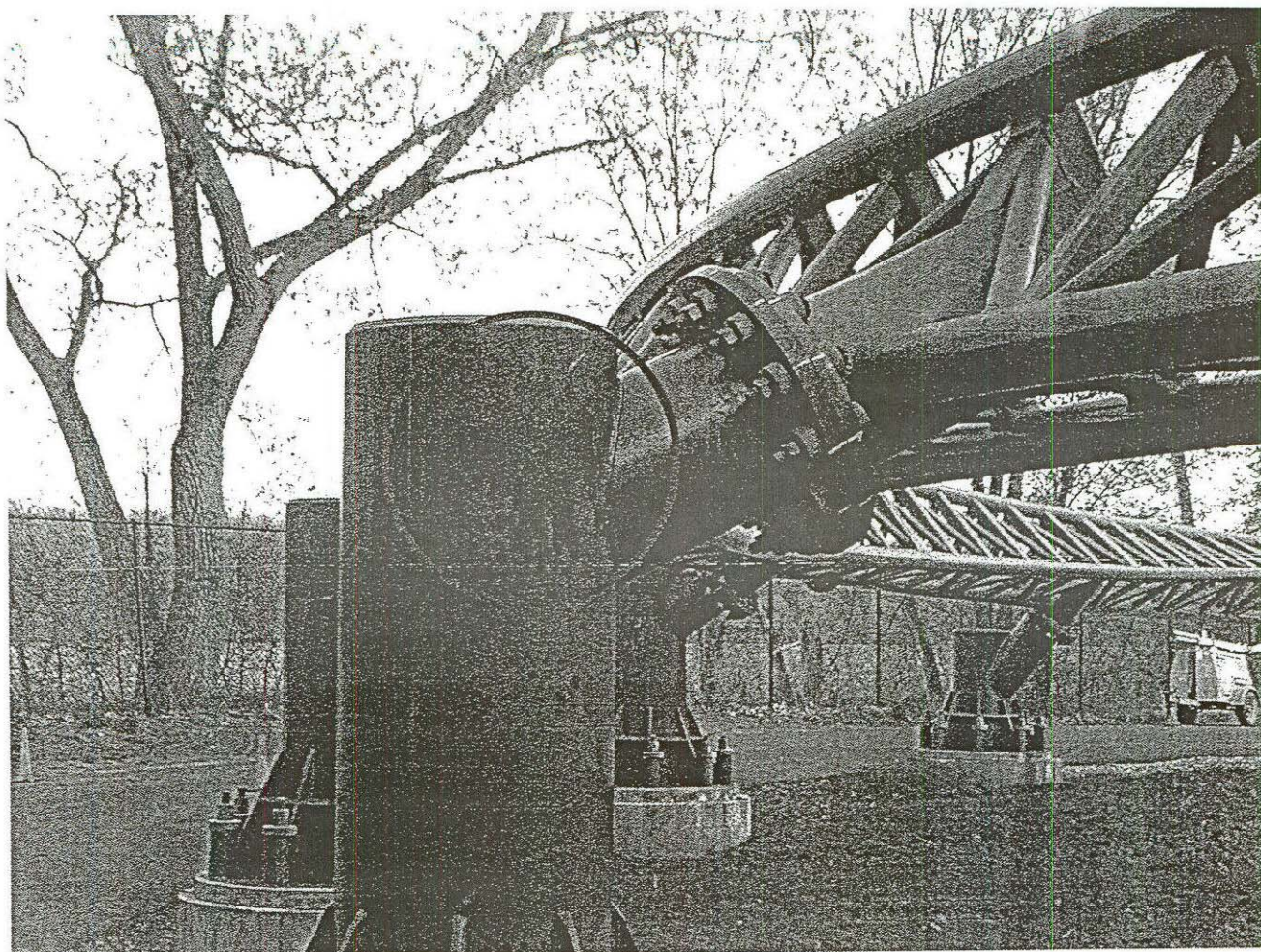
Photo #11 – Photo of location where victim struck #6 support column
